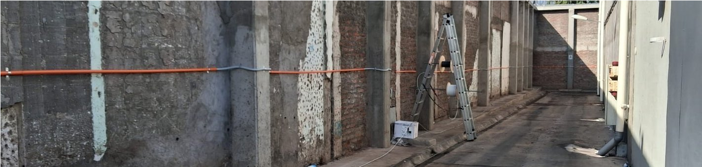
WALLALERT SENSOR CABLE INSTALLED ALONG A BANK FACILITY PERIMETER WALL. CUSTOMER IDENTITY WITHHELD.
