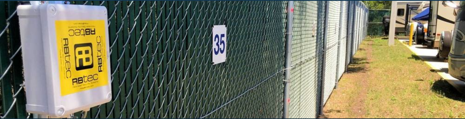
IRONCLAD SENSOR CABLE AND FIELD ENCLOSURE ON A CHAIN-LINK STORAGE PERIMETER. SITE AND CUSTOMER DETAILS WITHHELD.
