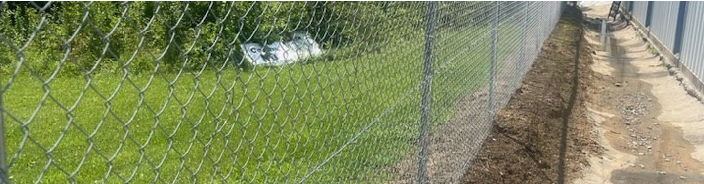
IRONCLAD SENSOR CABLE ON THE PERIMETER FENCE OF A SELF-STORAGE FACILITY. CUSTOMER IDENTITY WITHHELD.
