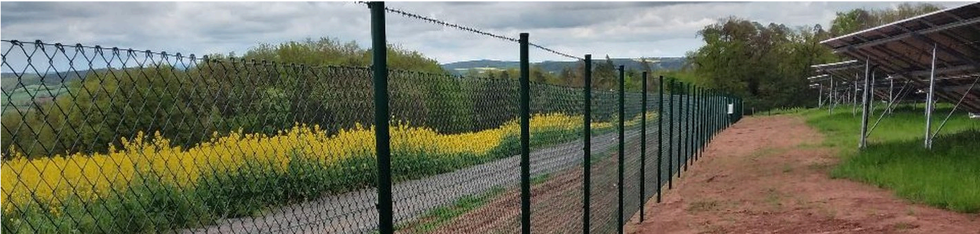
MICALERT SENSOR CABLE ON A SOLAR PARK PERIMETER FENCE. CUSTOMER IDENTITY WITHHELD.
