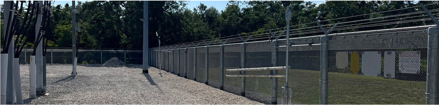
IRONCLAD-PROTECTED PERIMETER FENCE INSIDE THE SUBSTATION YARD. CUSTOMER IDENTITY WITHHELD.
